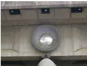
Metal reflectors on Kings Avenue Bridge (note pitting due to thrown rocks)
