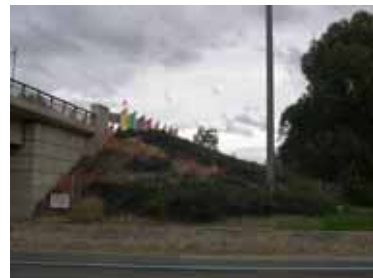
Approach to the bridge viewed from Bowen Drive, showing erosion
